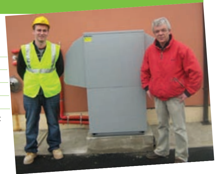
Dave Coleman of Pure Energy Technology Ltd and Joe Donovan beside Joe's new Dimplex LA11MS air-to-water heat pump.
